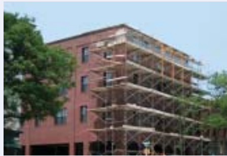
Casey Family Services will move its Waterbury, Vermont office to this newly renovated, 100-year-old building in downtown Winooski this fall.
